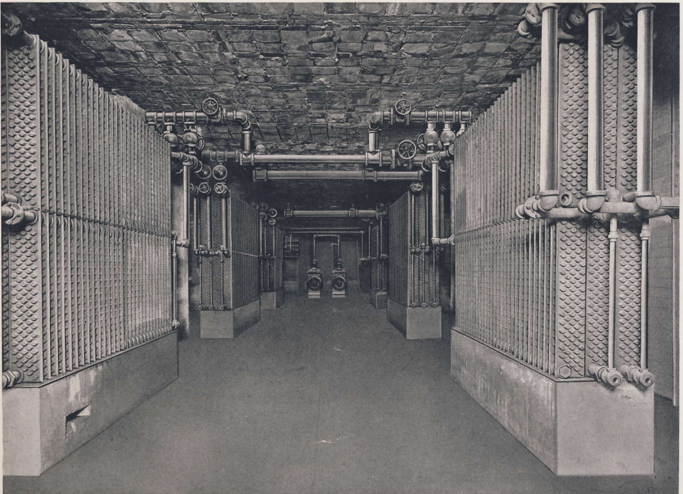
One of the two chambers of VENTO Heaters used in New Terminal Station of Chicago & Northwestern Railway in Chicago
