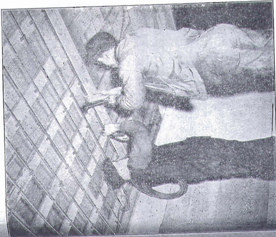
Fig. 7.—Showing method of installing copper tubing on ceiling. The copper tubing because of its great flexibility is easy to install on the ceiling while it is being uncoiled. Note how a board is being used to space the tubing evenly. Courtesy Chase Brass & Copper Co.
