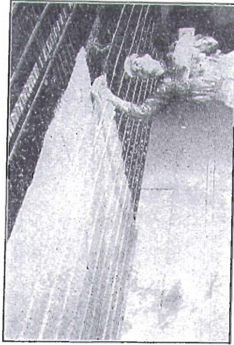
FIG. 8.—Showing application of first coat of gypsum plaster to ceiling. Other coats will give final cover of \frac{1}{4} inch over copper tube. Courtesy Chase Brass & Copper Co.
